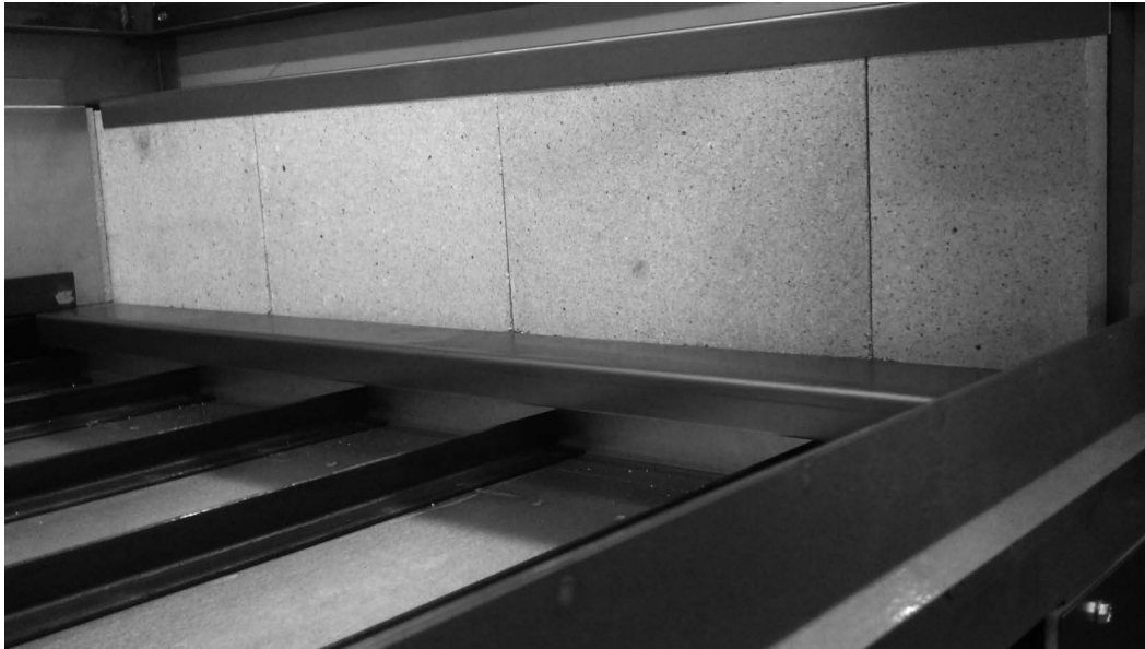
Bottom solid two piece deck on 14P-1. Metal covering removed from sides and back.
