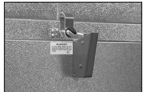
Roller Too High
