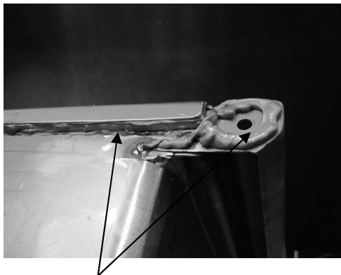
SEALANT APPLIED TO UNDERSIDE OF JBZ JOINT AND FACE OF THE END PLATE
