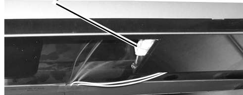
Wire Assembly Under BBLZ
