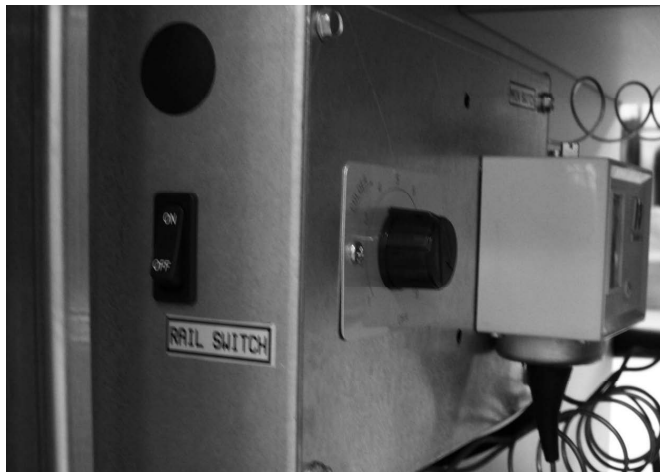
Figure 1 illustrates the electrical control box inside the mechanical compartment. The on/off switch for the rail is located on the front of the control box while the main on/off switch for the entire unit is located on the rear of the control box. The thermostat adjustment knob for the upper rail is located on the side of the control box.
