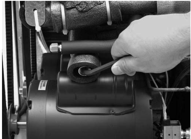
Figure 5-8 Hot Gas Bypass Adjustment
