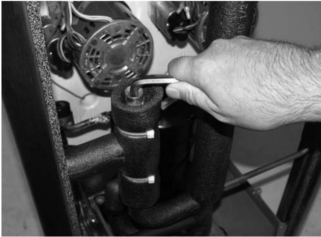
Figure 5-8 Hot Gas Bypass Adjustment
