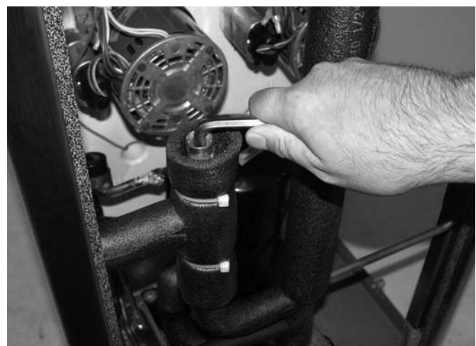
Figure 5-10 Hot Gas Bypass Adjustment
