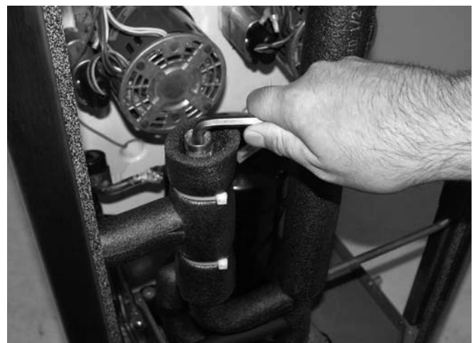
Figure 5-10 Hot Gas Bypass Adjustment
