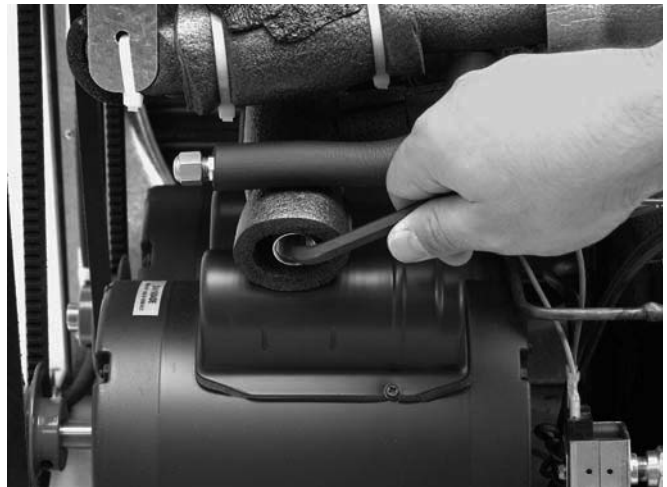
Figure 5-8 Hot Gas Bypass Adjustment
