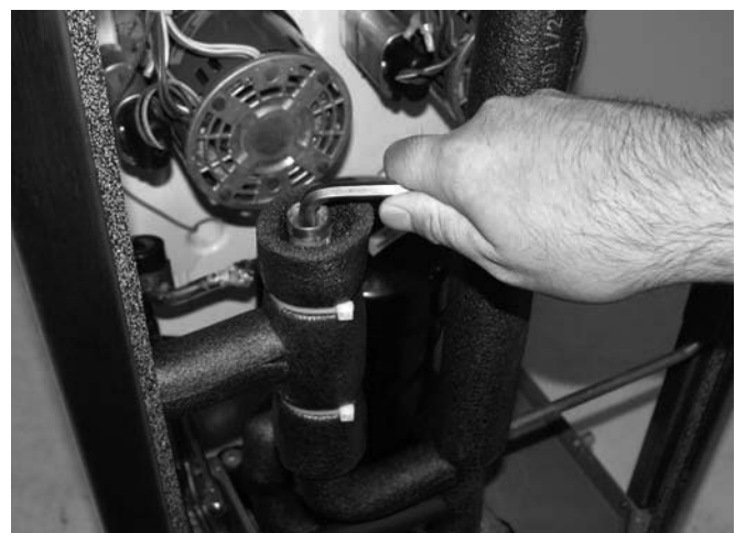
Figure 5-8 Hot Gas Bypass Adjustment
