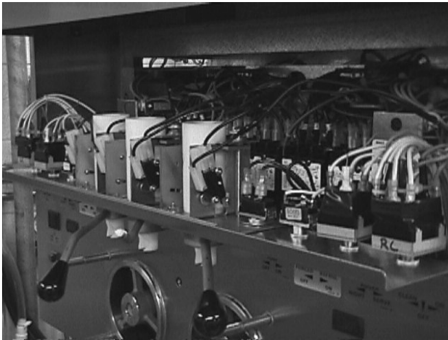
Figure 45. Front Electrical Box
