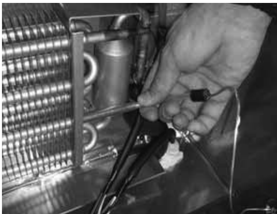
TEMPERATURE CONTROL & EVAPORATOR
