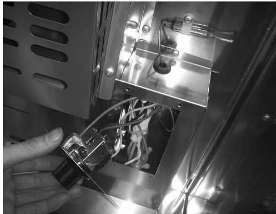
TEMPERATURE CONTROL & EVAPORATOR
